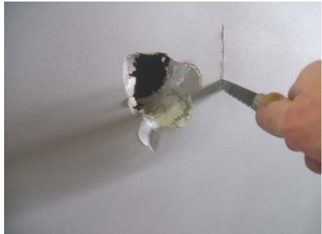
Figure 2. Square-Off Damaged Area
