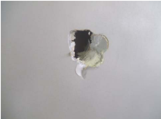
Figure 1. Damaged Gypsum Board
